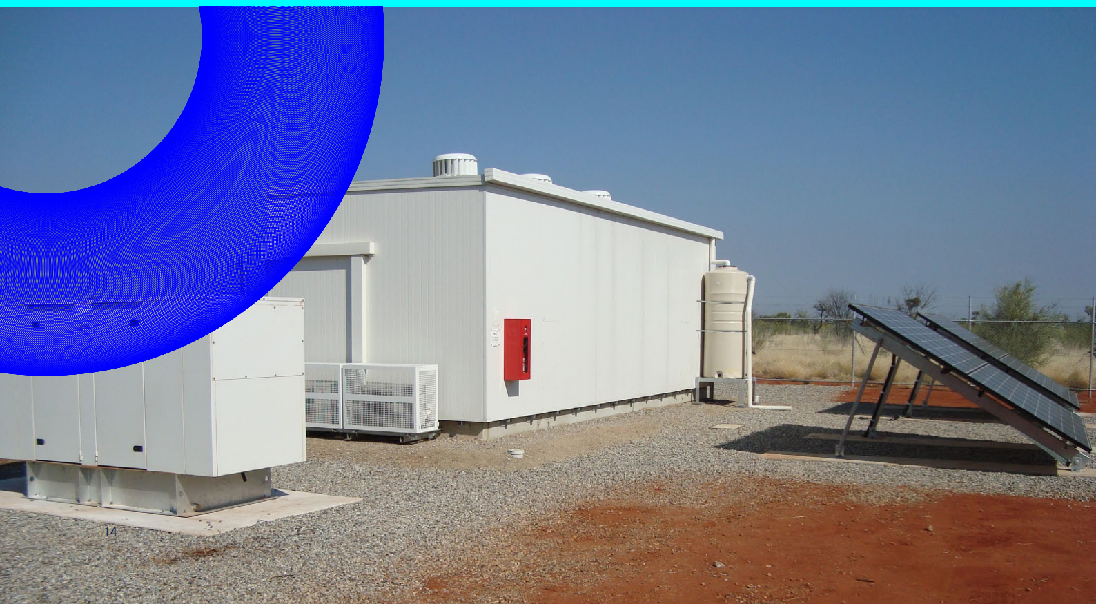
CEV with rain water tanks
